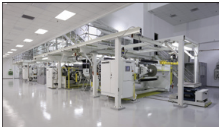
CLC's new line is equipped for multiple coating modes and quick changeovers.
